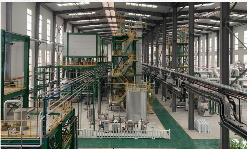
Real scene of CKB lithium battery recycling project
